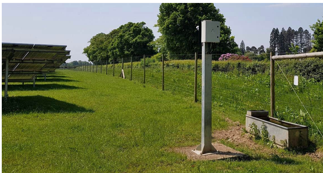
Figure 2-11: Metal CCTV pole and 'deer fence'
