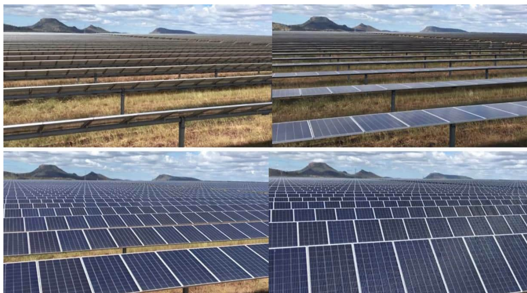
Figure 2-5: East-west single axis tracker system, finished array
