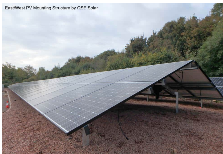
Figure 2-4: East-west facing fixed tilt modules, finished array
