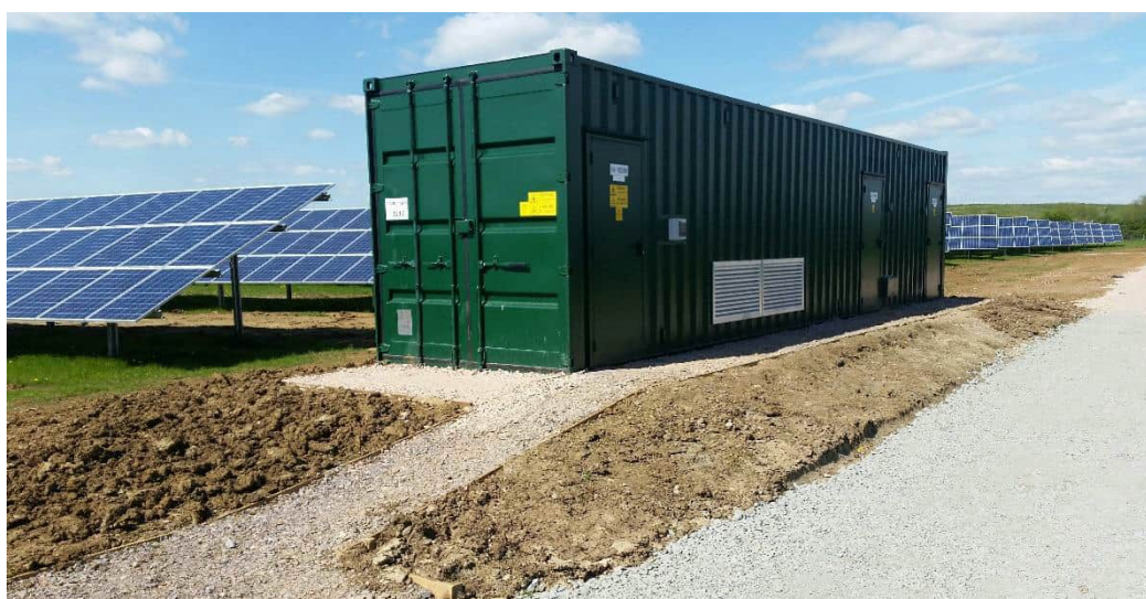
Figure 2-8: Example field substation
