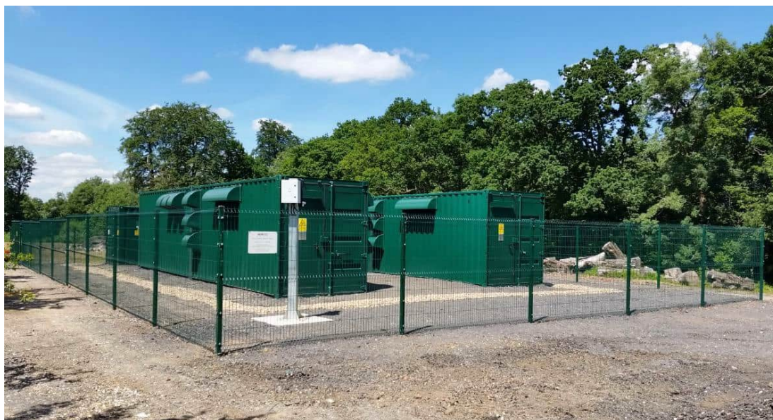
Figure 2-7: Typical central inverter
