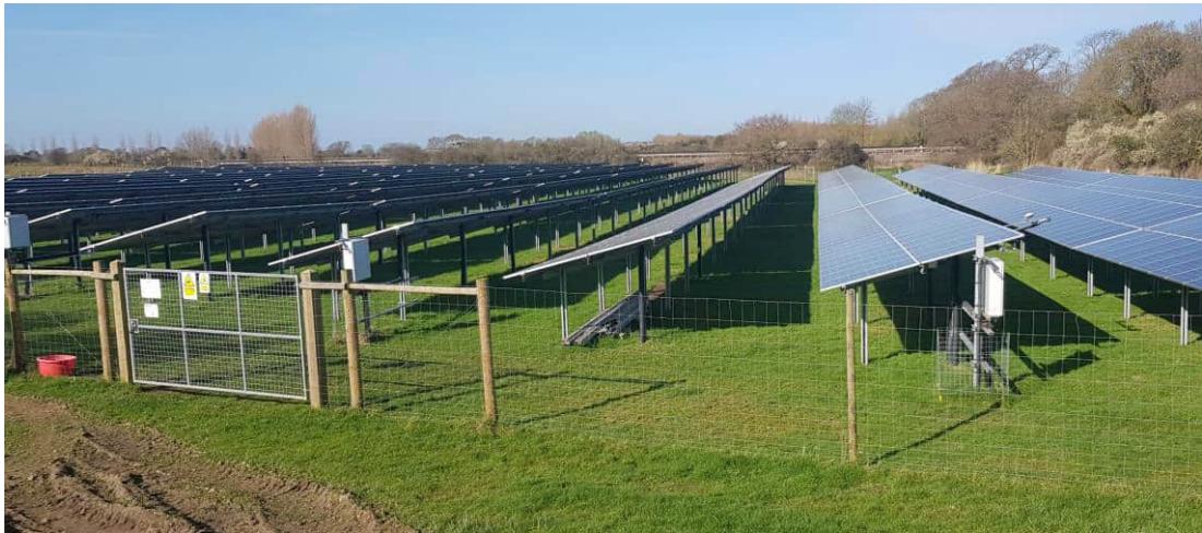
Figure 2-3: South-facing fixed tilt modules, finished array
